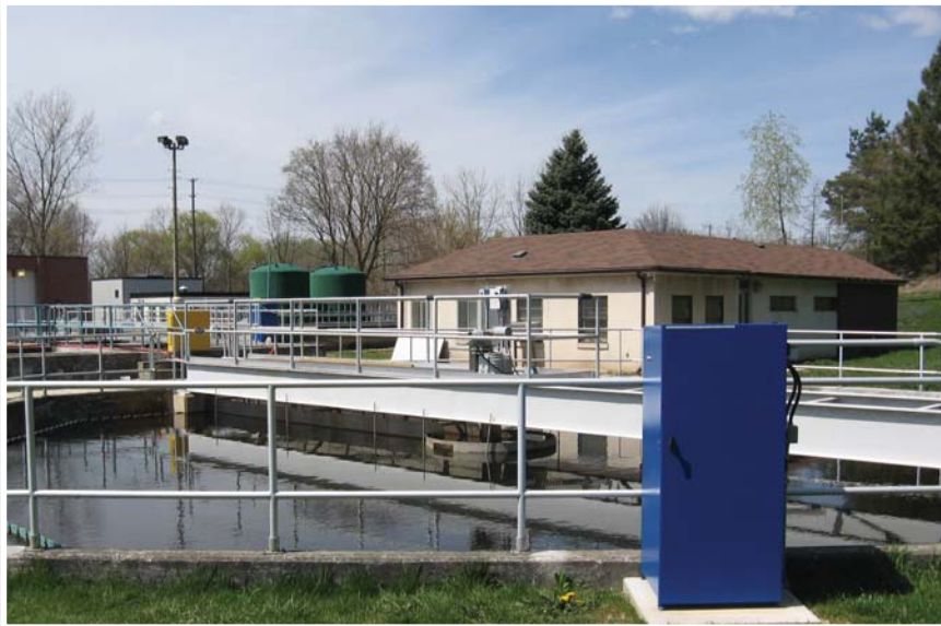
Final clarifier and effluent sampler.
