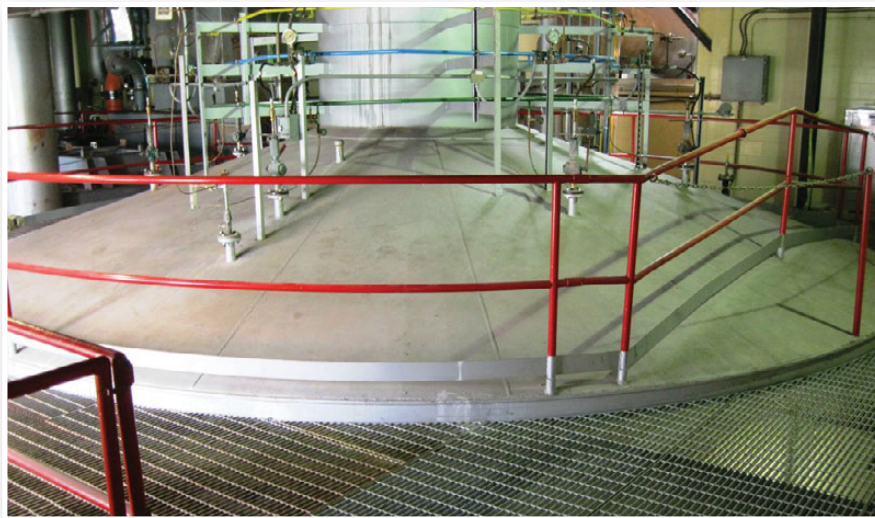
Top of the fluidized bed incinerator at Greenway Pollution Control Centre in London, Ontario.
