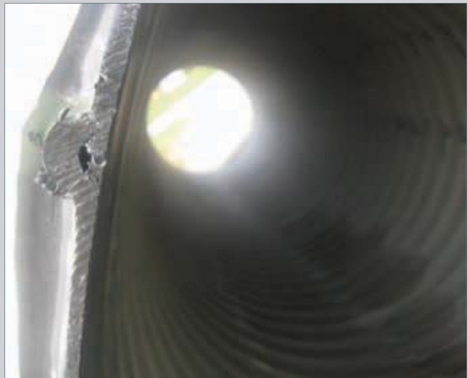
Figure 1: 5mm diameter channel on exterior of HDPE pipe
